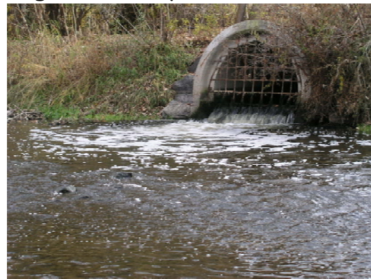
Effluent outfall point. Photo courtesy of City of Boise.
