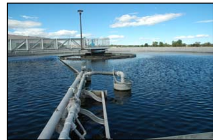
Secondary clarifier. Image courtesy of City of Boise
