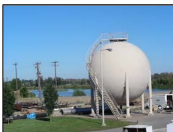
Gas Sphere. Image courtesy of City of Boise
